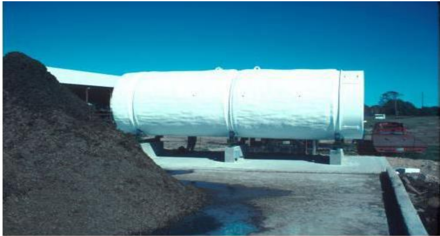
An example of in-vessel composting.
